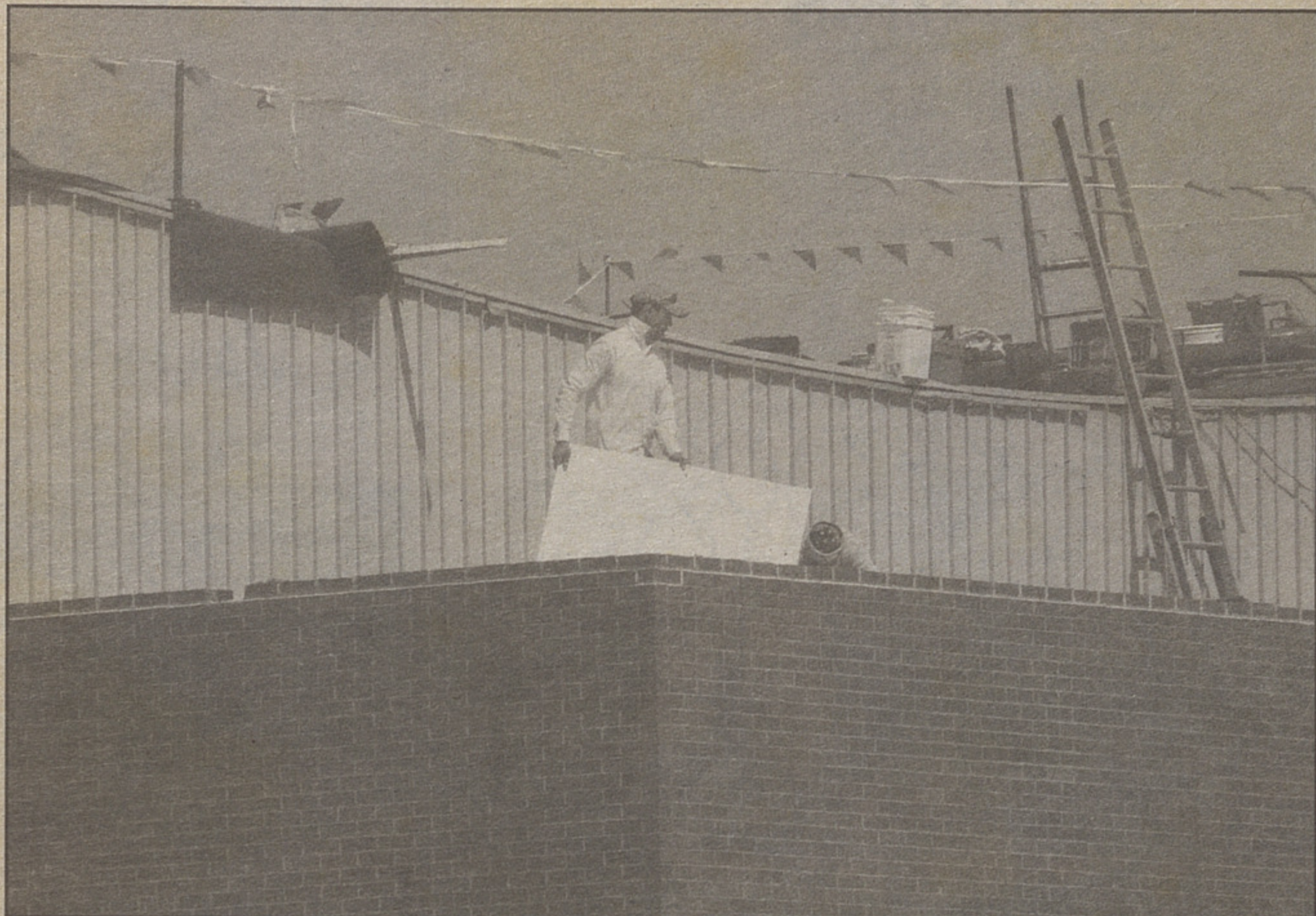
Superintendent Sandra Fellin said work to replace the Saucon Valley High School roof is progressing well. The million-dollar rubberized roof is being installed by J.M. Young & Sons and is expected to be finished this summer. Photo by Paul Bealer
